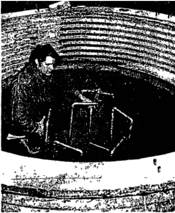
HEATING SYSTEM —Stanley Meyer begins installation of the heat exchanger in the storage cavity of the solar thermal electric power generation system he is building on Marlane Drive. A translucent silo-lens structure will be constructed above the storage cavity to collect sun rays.
